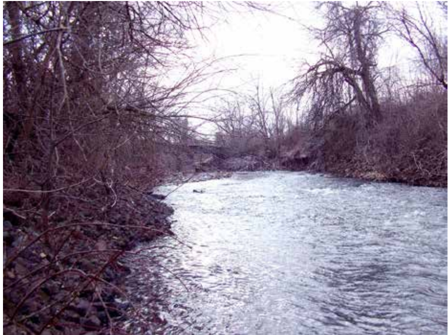
View upstream within terrace, showing steep banks and industrial rubbish.
